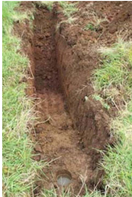
This is a typical test pit excavated for infiltration. Note that an infiltrometer was placed at the bottom of the pit.
